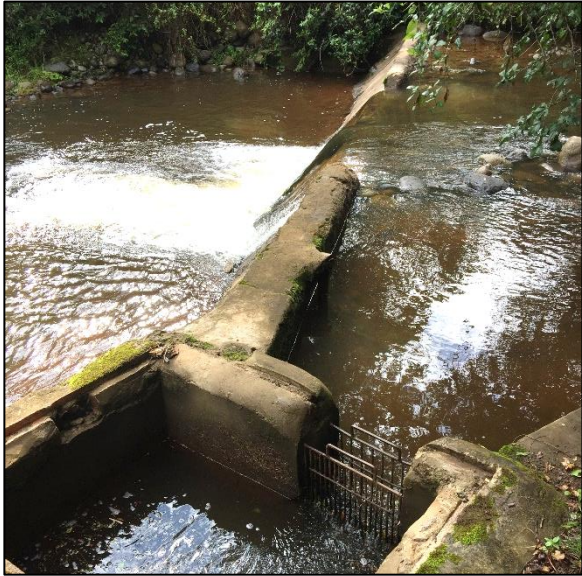
Figure 9: A river water intake for CWPs inside Nanyuki WRUA
